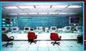
Subway dispatch center
