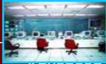
Subway dispatch center
